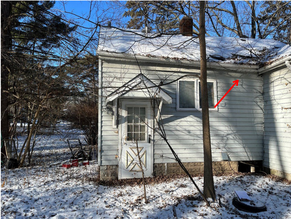
Photo 5 – Rear exterior wall. The left side of this wall is no longer providing support for the roof
