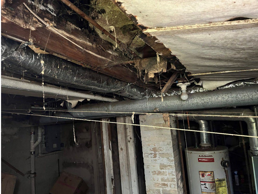
Photo 20 – Upper left appears to indicate rotted main level floor joist
