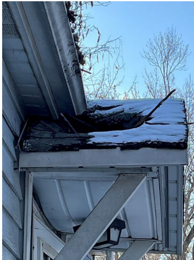
Photo 2 - Hole in the roof of the front canopy
