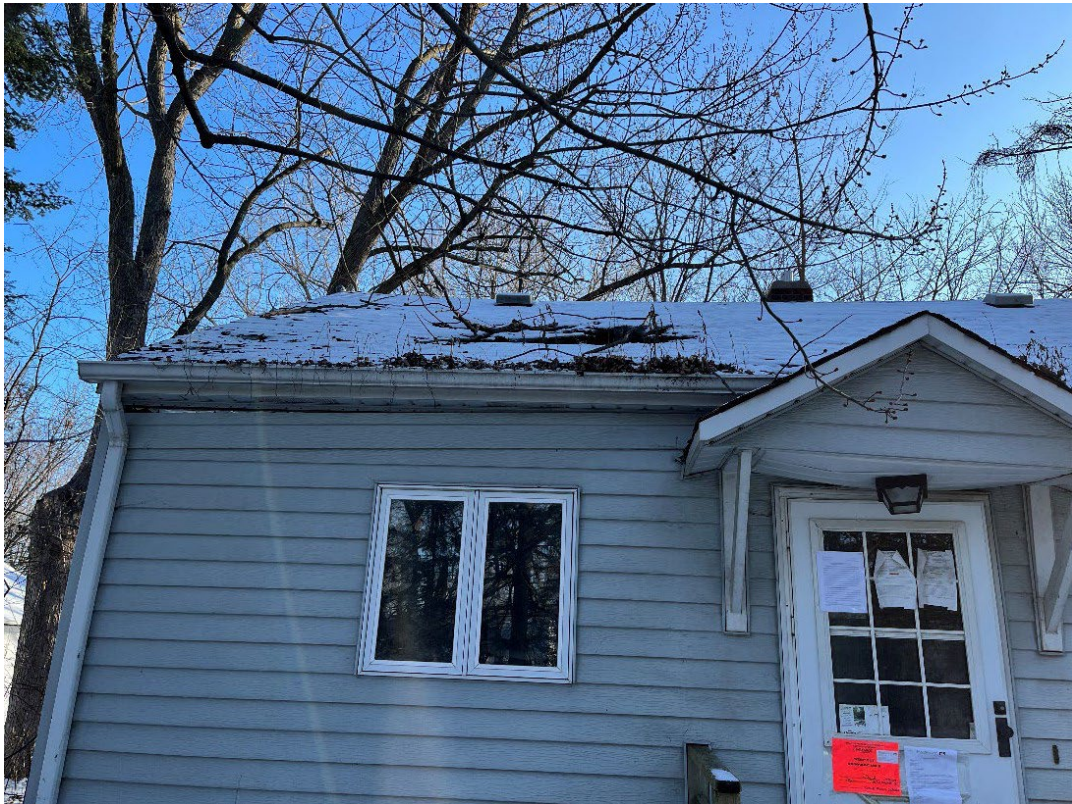
Photo 1 - Large hole in the roof on the front side of the house
