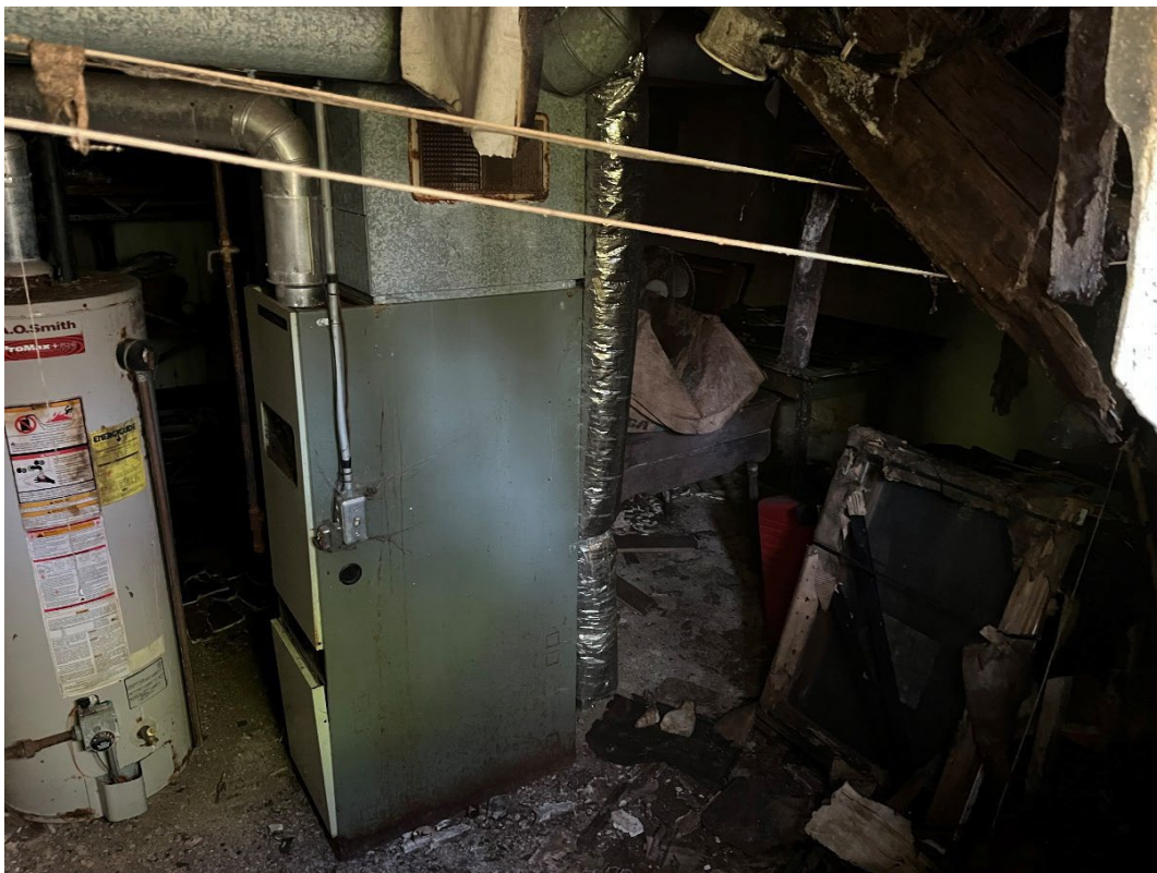
Photo 21 – Upper right appears to indicate some collapsed structure
