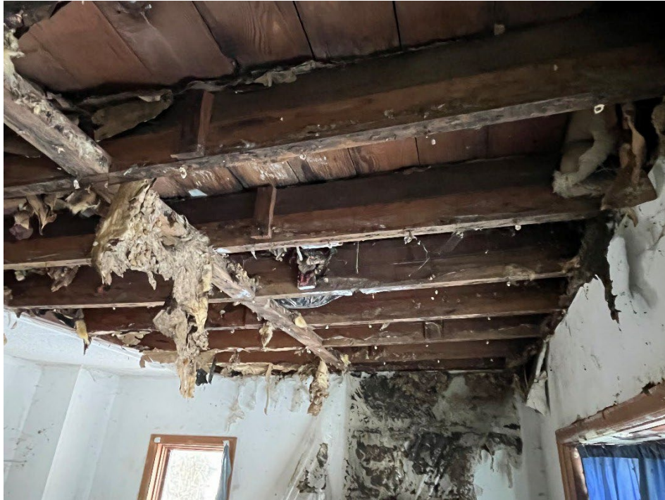
Photo 13 – Ceiling in the front living room has collapsed due to deterioration
