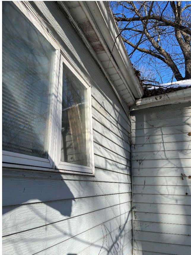
Photo 6 – Corner of the exterior wall showing the displacement in the roof
