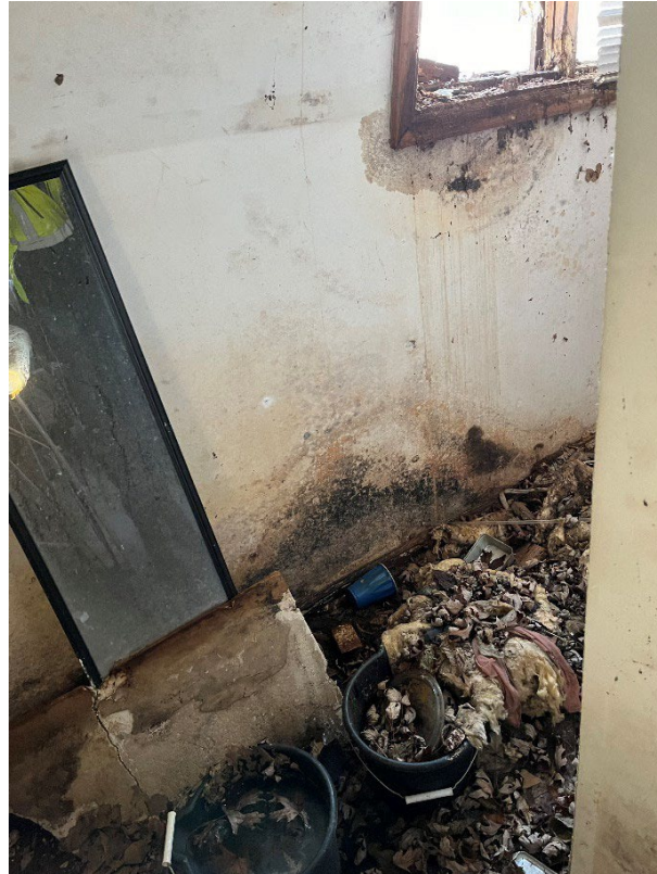
Photo 17 – Another photo of the sinking floor along the back wall
