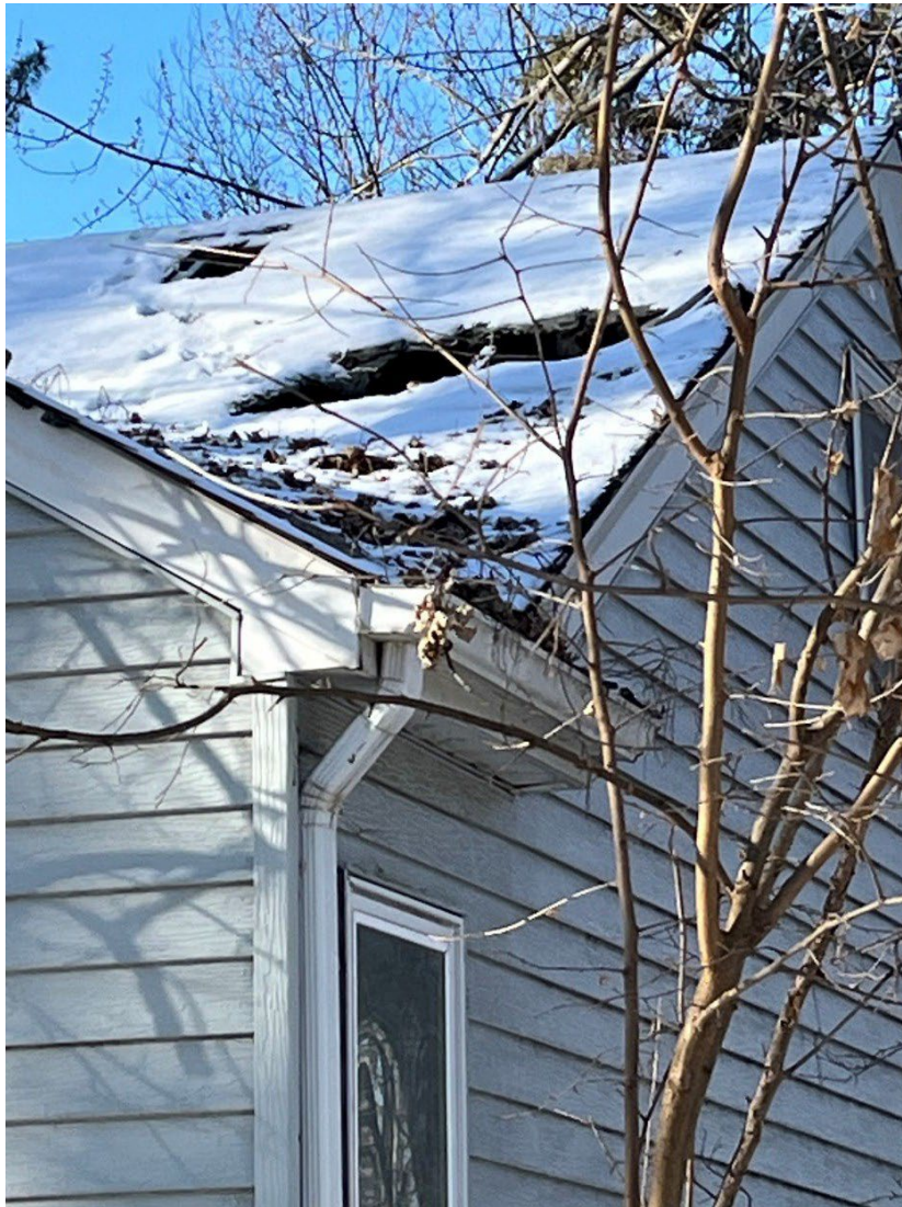
Photo 4 – Another hole in the roof at the rear of the house
