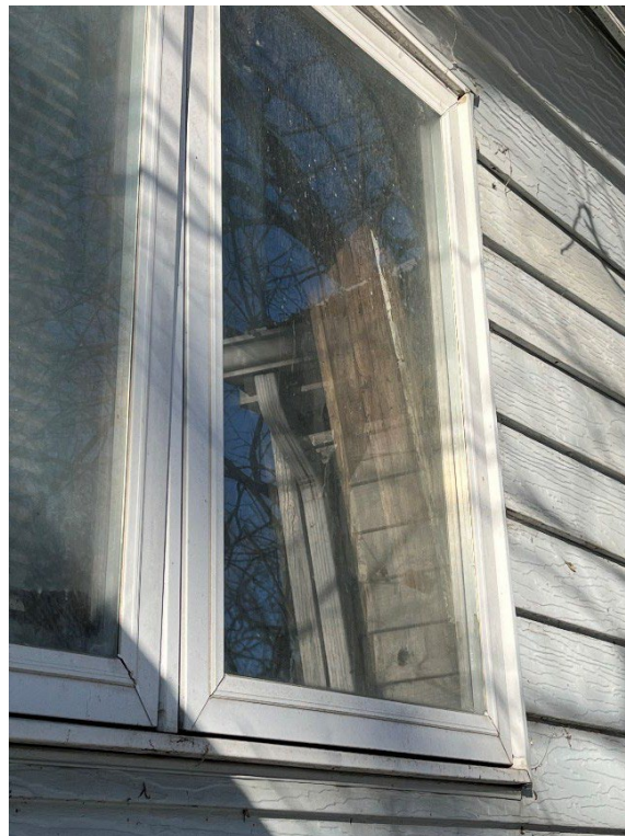
Photo 7 – Exterior wall is visible through window and is displaced and leaning inward
