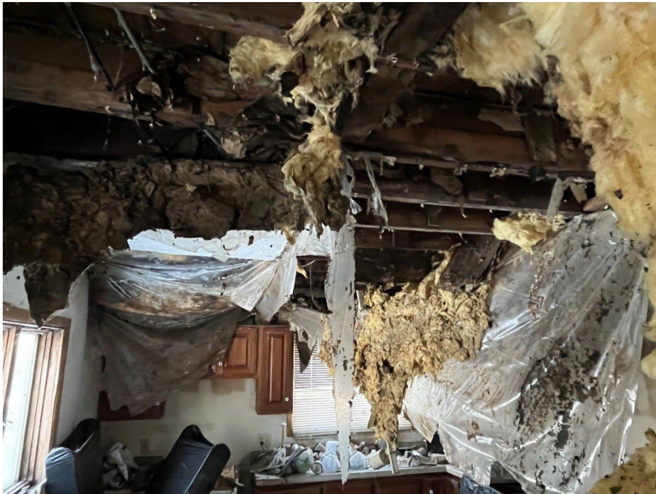
Photo 14 – Ceiling in the kitchen area has collapsed due to deterioration
