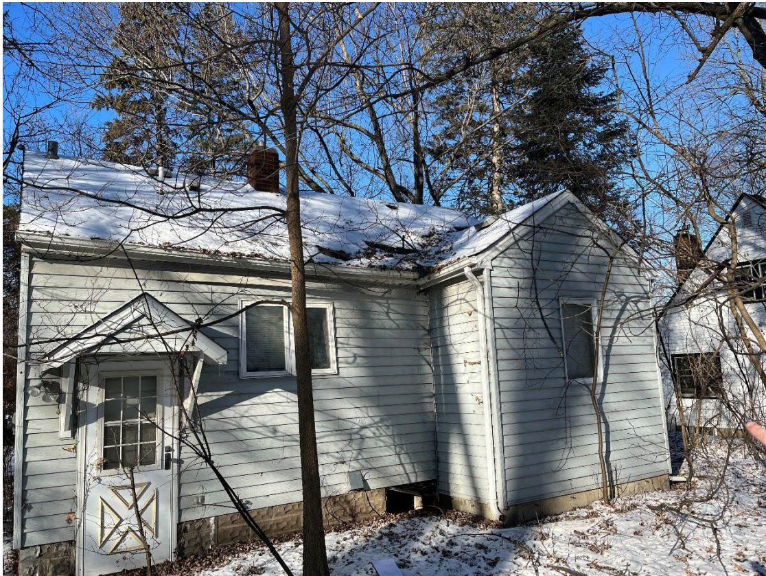
Photo 3 - Hole in the roof at the rear of the house
